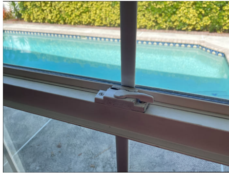
Locks were missing/damaged at family room.
