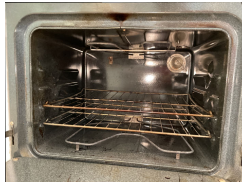
Oven was not functioning properly. No broiler. No Light.
