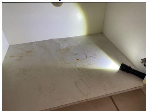
Dry stain(s) were visible under sink at hallway bathroom.
