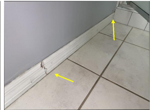
Wall at the exterior of shower enclosure was damaged at the primary bathroom.
