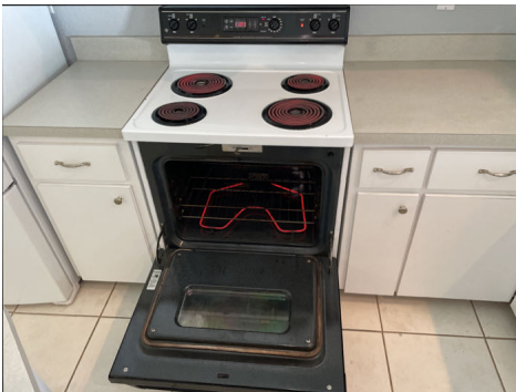
Oven light did not operate.
