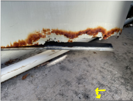
Moisture damage was visible at the door and/or door jamb.
