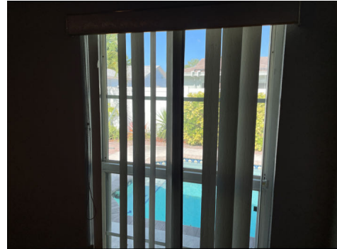
Window tension spring(s) were damaged at multiple locations.
