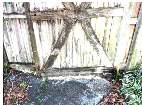
Gate(s) were damaged.
