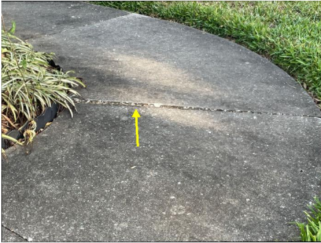
Driveway/Walkway surface was raised/settled. Trip hazard noted.
