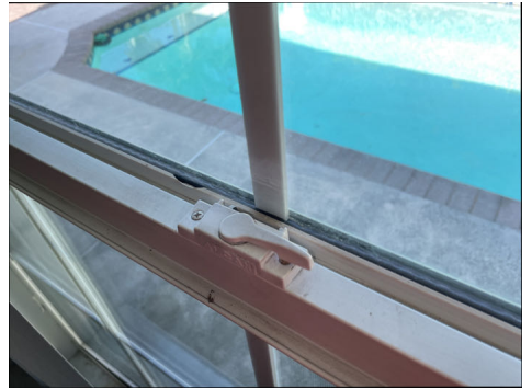
Locks were missing/damaged at family room.
