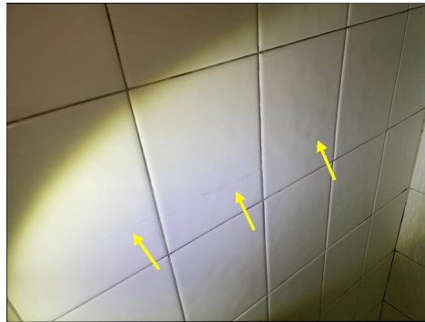
Cracked tiles were visible at primary bathroom.
