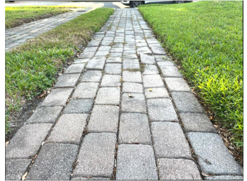
Driveway/Walkway surface was raised/settled. Trip hazard noted.
