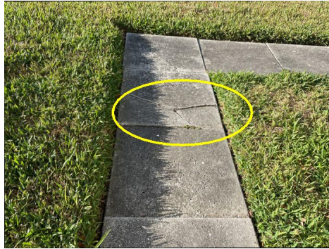
Walkway had large and displaced crack(s) visible.
