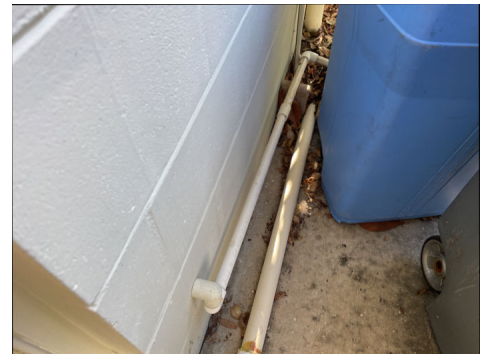
Proper trap was not installed at the condensation line.
