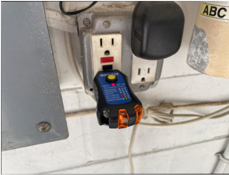
GFCI (Ground Fault Circuit Interrupter) outlet(s) was damaged at garage outlets.
