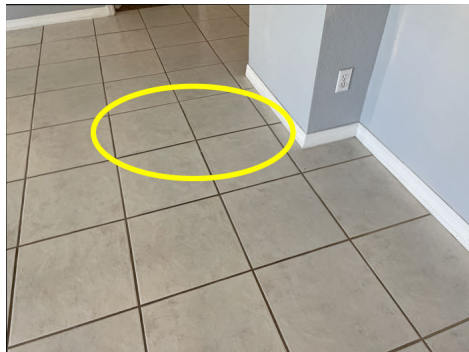
Tile flooring was disbonded at family room. Hollow sound can be heard when the flooring was tapped.
