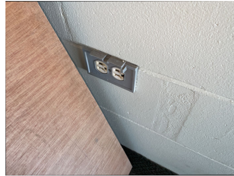
Weatherproof covers were damaged/missing at exterior outlet(s).
