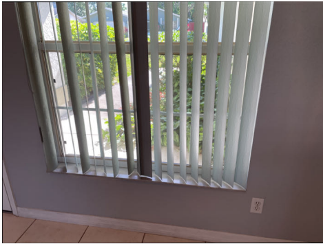
Window tension spring(s) were damaged at kitchen.
