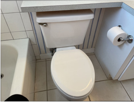
Toilet was loose at the floor at all bathrooms.
