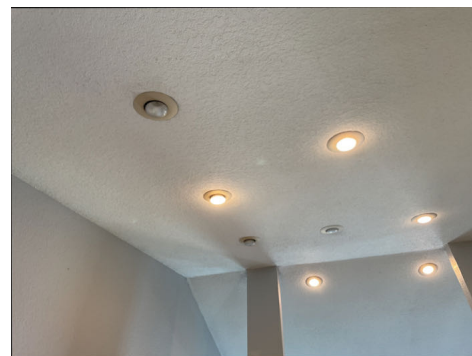
Light(s) were tested and not operational at multiple locations.
