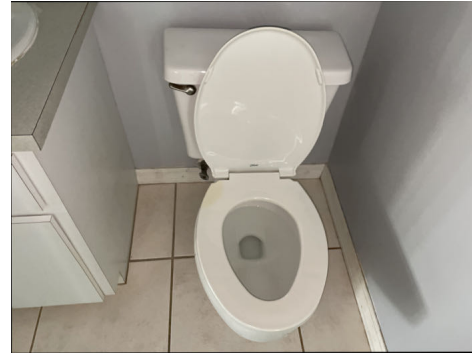
Toilet was loose at the floor at all bathrooms.
