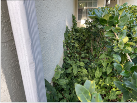
Landscaping and vegetation was poorly maintained and overgrown.
