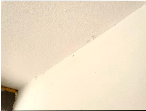
Ceiling seam separation was visible.
