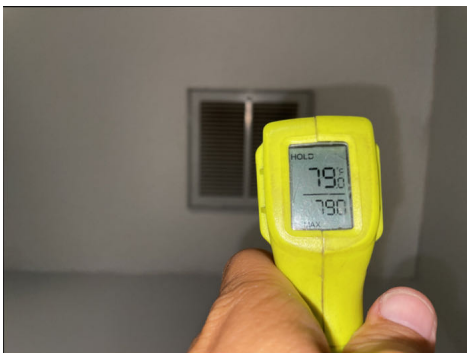
Return air temperature
