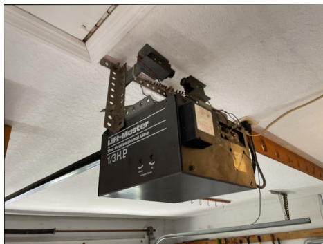
Electronic eye safety feature did not operate when tested.
