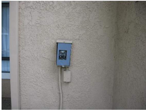
Heater/AC - Disconnect Box
