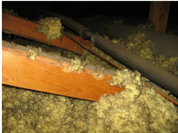
Heating/AC - Refrigerant Lines
