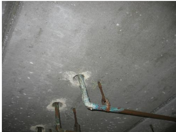
Sub Parking Area - Plumbing
