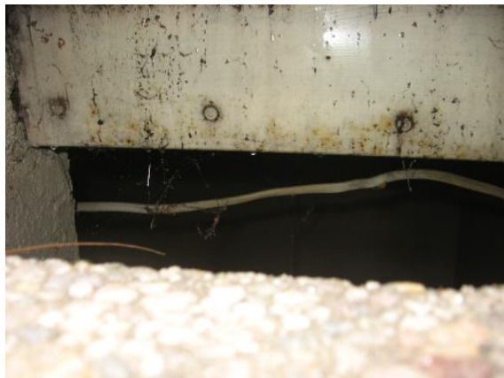
Grounds - Electrical Under Stairs
