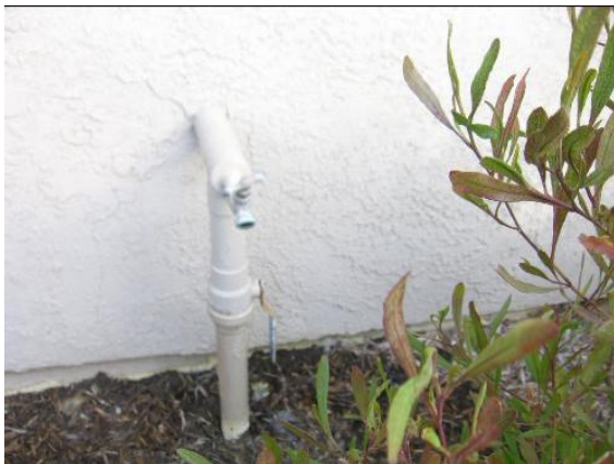
Grounds - Water Shut-off Valve
