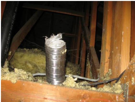
Laundry - Dryer Vent
