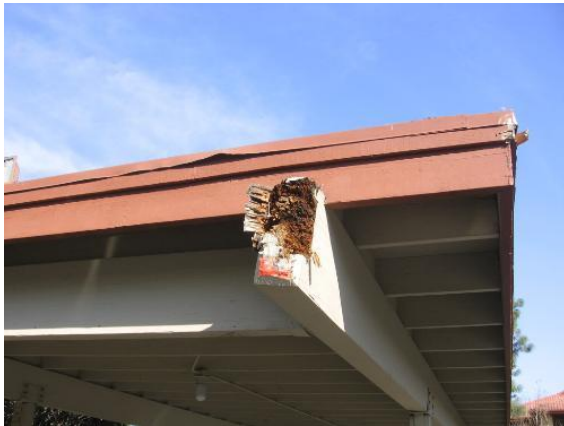
Car Port - Damaged Wood
