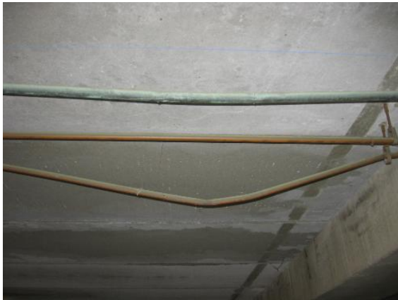
Sub Parking Area - Plumbing
