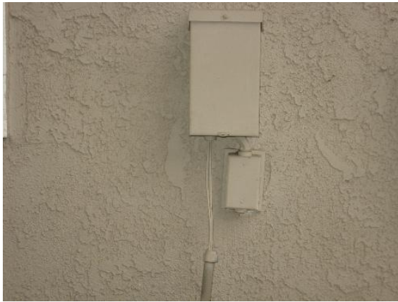
Heater/AC - Electrical Disconnect Box
