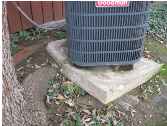
Heating - Condensor Base
