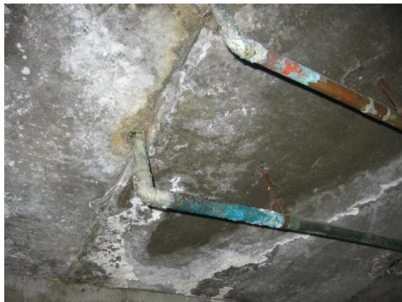
Sub Parking Area - Plumbing
