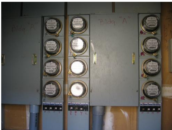
Electrical - Service Panel
