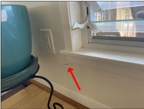
Minor cosmetic defects and damages at walls.
