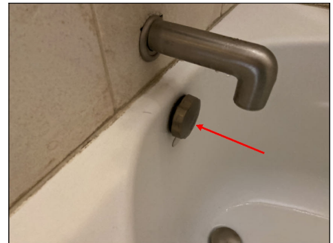
Loose tub overflow drain cap. Repair or replace as needed. (Blue) Location: guest bathroom.
