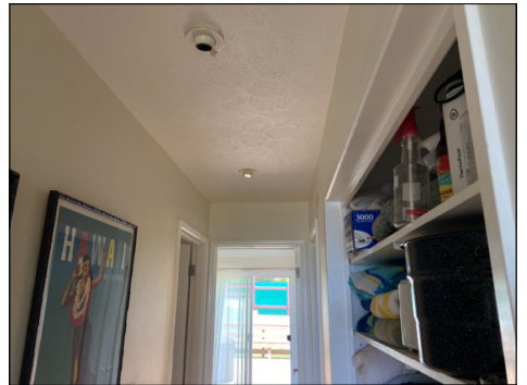
Smoke detectors not present. Recommend installing at currently required locations. (Red)
