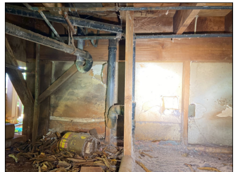
Damage to drywall on foundation side of wall behind the washer and dryer units. Evaluate. Repair or replace as needed. (Blue)
