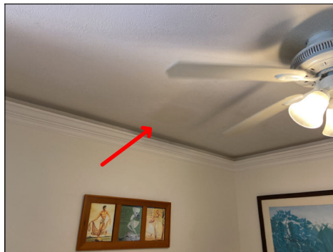
Discoloration or defects at ceilings. Normal moisture levels at time of inspection. Location: guest bathroom.
