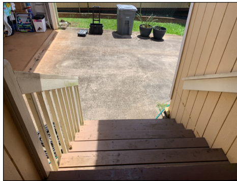
Current safety standards indicate that stairs with 4 or more risers should be equipped with a safety rail and graspable handrail. Update as needed. (Purple)
