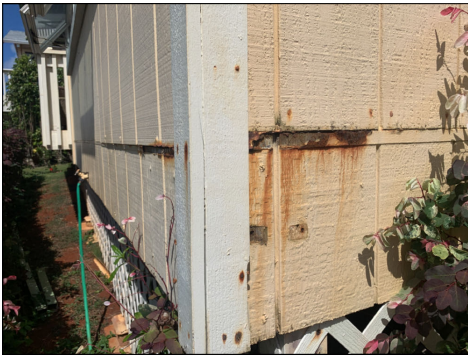
Corrosion at wall flashing. Repair or replace as needed. (Blue) Location: Photo location at front right of home. Condition exists at a few locations around the home.
