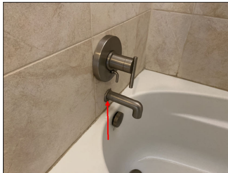
Seal tub spout to wall to prevent moisture intrusion. (Blue) Location: guest bathroom.
