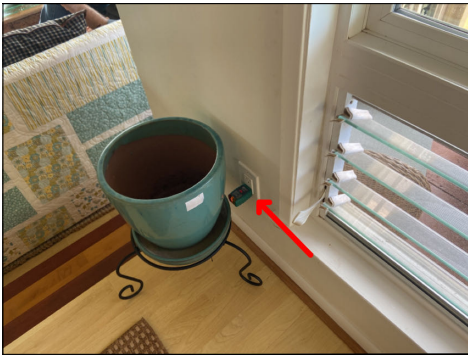
Outlet tester indicates the outlet was not grounded. Repair, replace or update as needed. (Red) Location: dining area.
