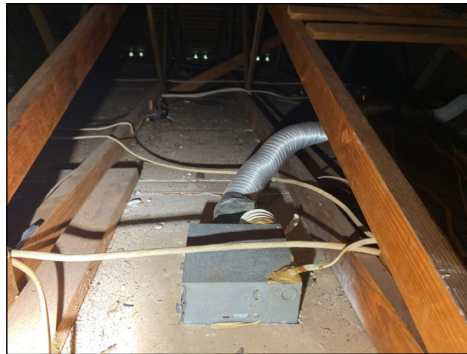
Bathroom exhaust fan(s) were not connected to the exterior venting. Repair. (Blue) Location: master bathroom.
