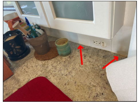
Cracked grout or missing/damaged sealant. Seal to prevent moisture intrusion. (Blue) Location: kitchen backsplash.
