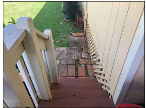
Current safety standards indicate that stairs with 4 or more risers should be equipped with a safety rail and graspable handrail. Update as needed. (Purple)
