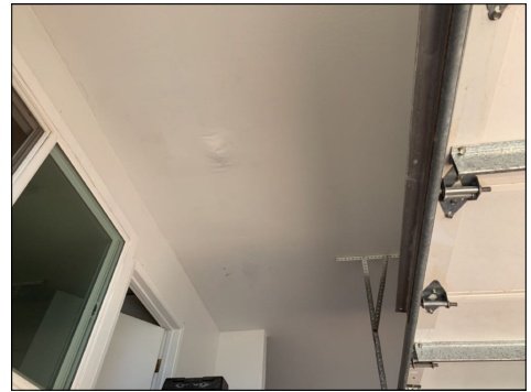
Drywall at garage was damaged due to solar hot water penetrations. Repaired or replace as needed. (Blue)
