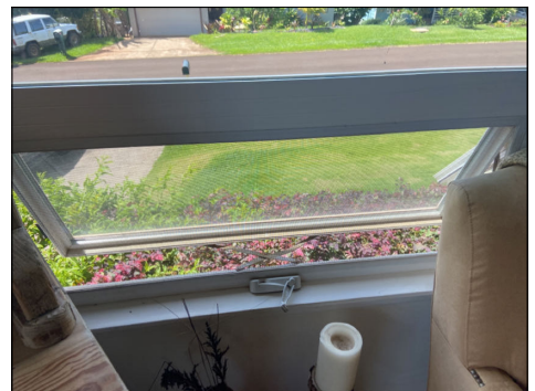
Window(s) did not operate properly. Repair as needed. (Blue) Location: living room.
