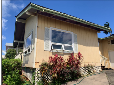
Missing downspout in the rain gutters were not properly secured. Repair or replace as needed. (Red) Location: right side of the home.
