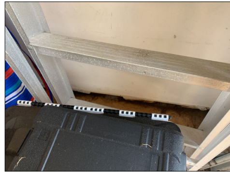
Damaged wood sill plates at right side of garage wall. Indications of moisture intrusion from water drainage. Limited view and accessibility due to personal belongings. Evaluate. Repair or replace components as needed. (Red)
