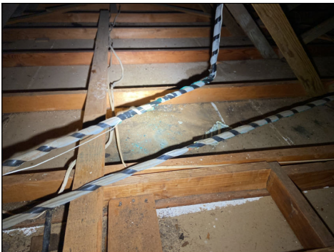
Drywall at garage was damaged due to solar hot water penetrations. Repaired or replace as needed. (Blue)
