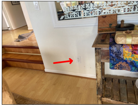
Loose outlets. Tighten. (Red) Location: living room.
