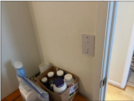
Flicker switch junction box appeared to be abandoned. Location: guest bedroom.
