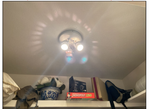
Replace dead or missing light bulbs. Test fixtures for proper operation. (Blue) Location: master bathroom closet.
