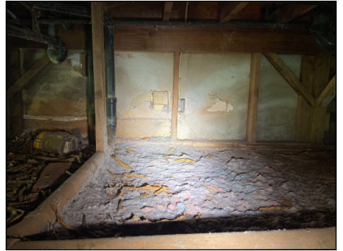
Large amount of lint at foundation area. Fire hazard. Remove lint and direct dryer duct to the perimeter of the home. (Red)
