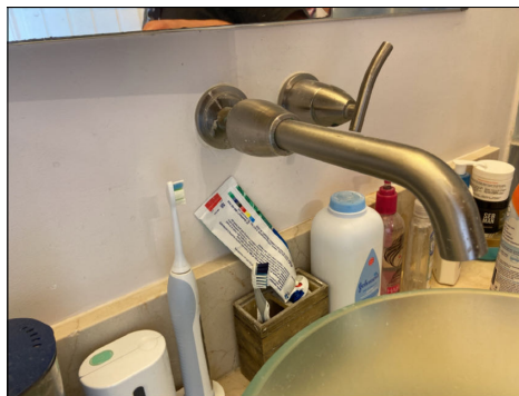
Loose sink wall cover hardware. Repair or replace as needed. (Blue) Location: master bathroom.
