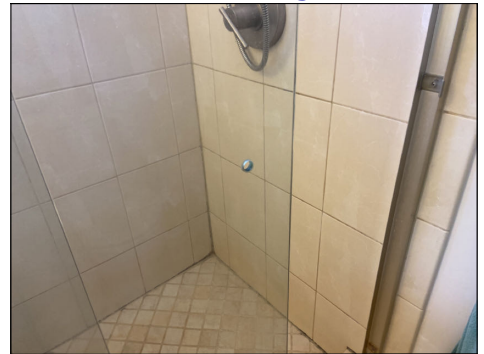
Missing sliding shower door handle. Install. (Blue) Location: master bathroom.
