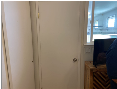
Door from garage to home did not meet the requirements for fire separation between garages and homes. Replace. (Red)
