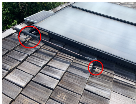
Solar water heating roof penetrations did not appear to be adequately sealed. Indications of a leak with damaged drywall at the garage ceiling. Repair or replace components as needed. (Red)
