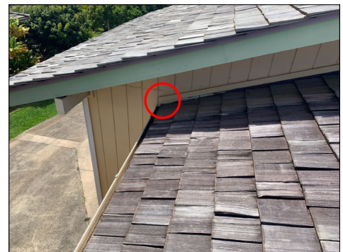
Kickout flashings were missing where the wall continued past the roof. Kick out flashing divert waters away from the structure and helps prevent damage to walls. There were no significant damages to the siding at this location however installation recommended time the roof is replaced. (Blue) Location: right side of home.
