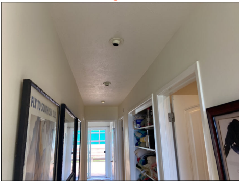
Replace dead or missing light bulbs. Test fixtures for proper operation. (Blue) Location: hallway.
