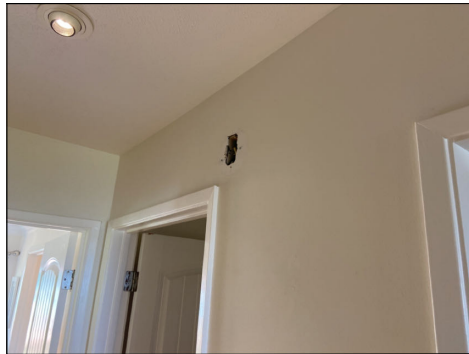
Install covers at open junction boxes. (Red)
