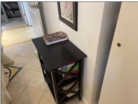
Minor cosmetic defects and damages at walls.
