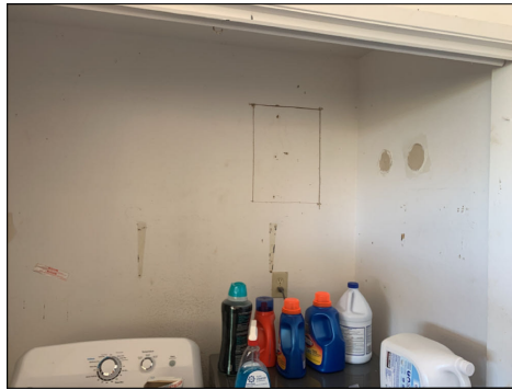
Access cut into wall at garage. Master bathroom shower on other side.
