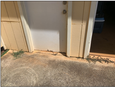
Minor to moderate damage to door(s). Maintain or repair as needed. (Blue) Location: front of garage.
