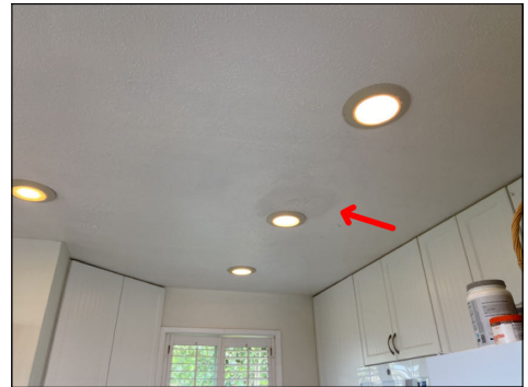
Discoloration or defects at ceilings. Normal moisture levels at time of inspection. Location: kitchen.
