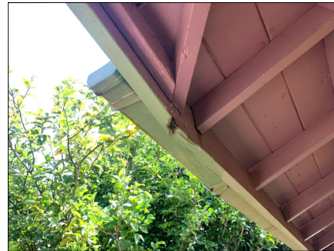
Damaged fascia/eaves. Evaluate and repair to prevent further damage. (Red) Location: rear of garage at rear lanai.
