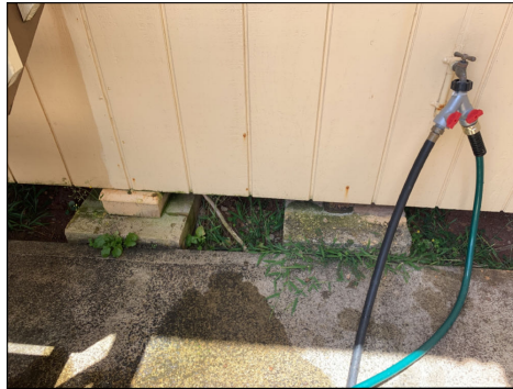
Damaged wood foundation post. Repair or replace as needed. (Red) Location: right side of home adjacent to main entry deck.
