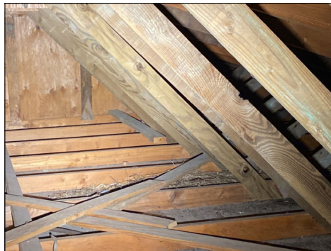
Bird nest(s) was observed in attic. Remove. (Blue)
