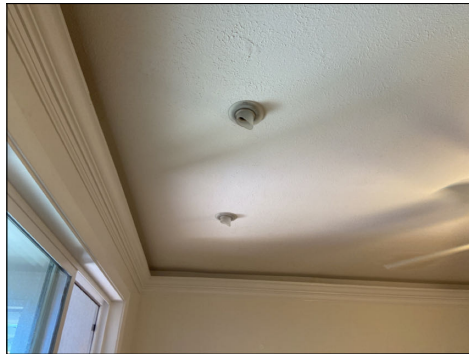
Replace dead or missing light bulbs. Test fixtures for proper operation. (Blue) Location: guest bedroom.
