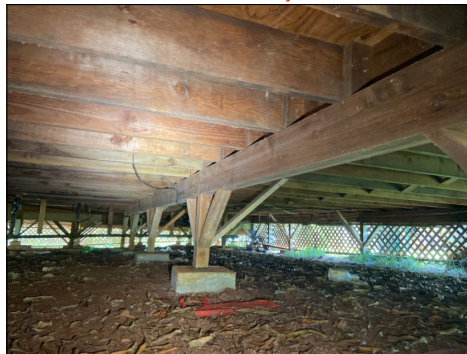
Foundation type - Raised foundation(s) inspected by walking or crawling under the home or structure(s) and/or remote control car with camera. Concrete piers, Wood posts, Floor system: 4X wood beams and 4 X wood joist, Plywood over floor joists.
