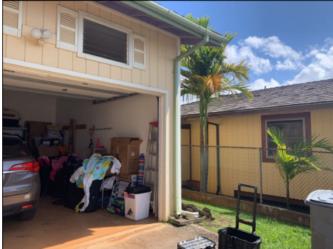
Rain gutter materials - Plastic.
