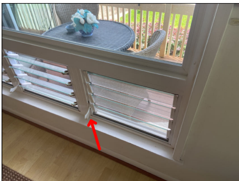
Missing, damaged or corroded window hardware observed. Repair or replace as needed. (Blue) Location: dining area.
