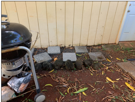
Soil/gravel/vegetation in contact with siding/trim components. The condition of the wall inside the garage was not clearly visible due to personal belongings. Evaluate the condition of the wall and repair the grade to prevent further damage. (Red) Location: rear of garage.
