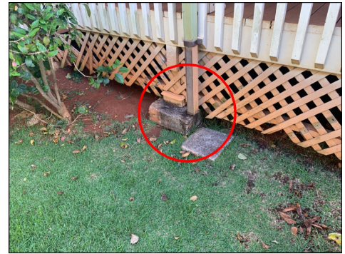
Rain gutter downspout discharges near deck foundation pier. Direct rain gutter discharge away from foundation components. Minor to moderate soil loss at deck foundation pier. (Red) Evaluate. Repair or replace as needed.
