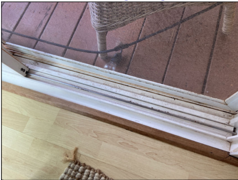
Corrosion common to our climate at sliding screen(s). Repair or replace as needed. (Blue) Location: living room.
