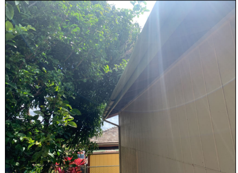
Disconnected rain gutter. Repair. (Red) Location: rear of garage.
