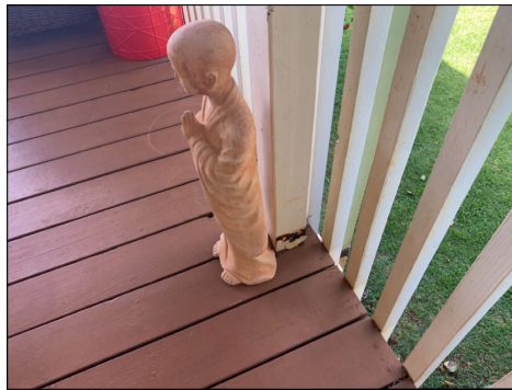
Corrosion at post base. Replace. (Blue) Location: front lanai.
