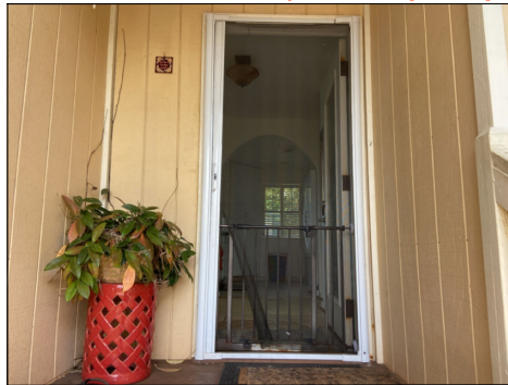
Damaged screen at screen door(s). Repair as needed. (Blue) Location: front door.
