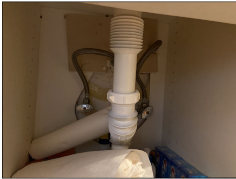
Flexible drain lines are subject to clogs and cracks. Replace with standard materials. (Blue) Location: master bathroom.
