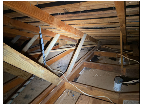
Insulation not present. The lack of insulation is not considered a defect in Hawaii.
