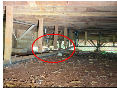
The bracing/strapping at drain lines at foundation area was corroded and/or not present to maintain proper slope of the drain line. Repair or replace as needed. (Red)
