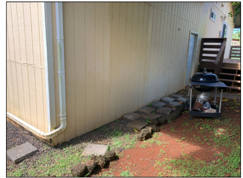
Damage siding and trim. Repair or replace as needed. (Blue) Location: rear of garage.
