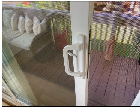
Loose slider door handle. Adjust or repair as needed. (Blue) Location: dining area.
