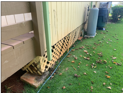
The roof drainage system channels water away from the foundation. Water from the roof can raise the moisture content in soil near the foundation which can affect its ability to support the structure and may cause foundation damage. Direct rain gutter drainage away from foundation components to prevent damage. (Red)
