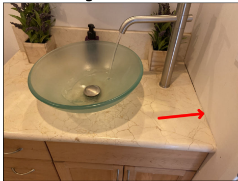
Cracked grout or missing/damaged sealant. Seal to prevent moisture intrusion. (Blue) Location: guest bathroom.
