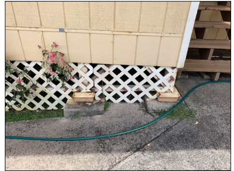
Damaged wood foundation post. Repair or replace as needed. (Red) Location: left side of home adjacent to main entry deck.
