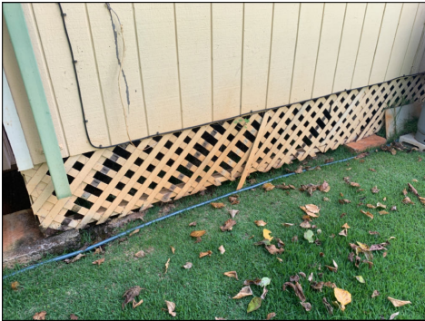
Damaged lattice foundation skirting got a few locations around the house. Repair or replace as needed.
