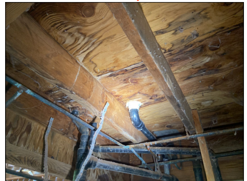
Stains or minor water damage at sub-floor. Normal moisture levels at time of inspection. Location: below master bathroom.
