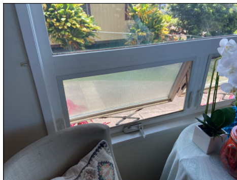
Window(s) did not operate properly. Repair as needed. (Blue) Location: living room.
